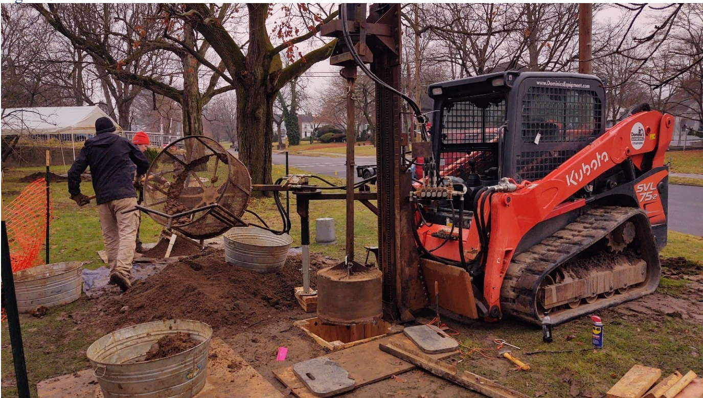
Deep testing through a wooden trench box as part of the Phase I Archaeology for the Pittston Bridge Replacement Project in West Pittston, Pennsylvania in January 2023.
